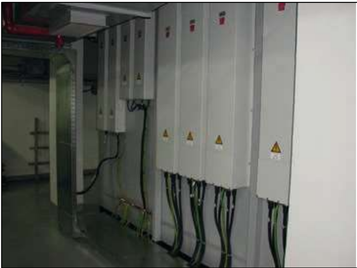
Filter elements outside IT-room
