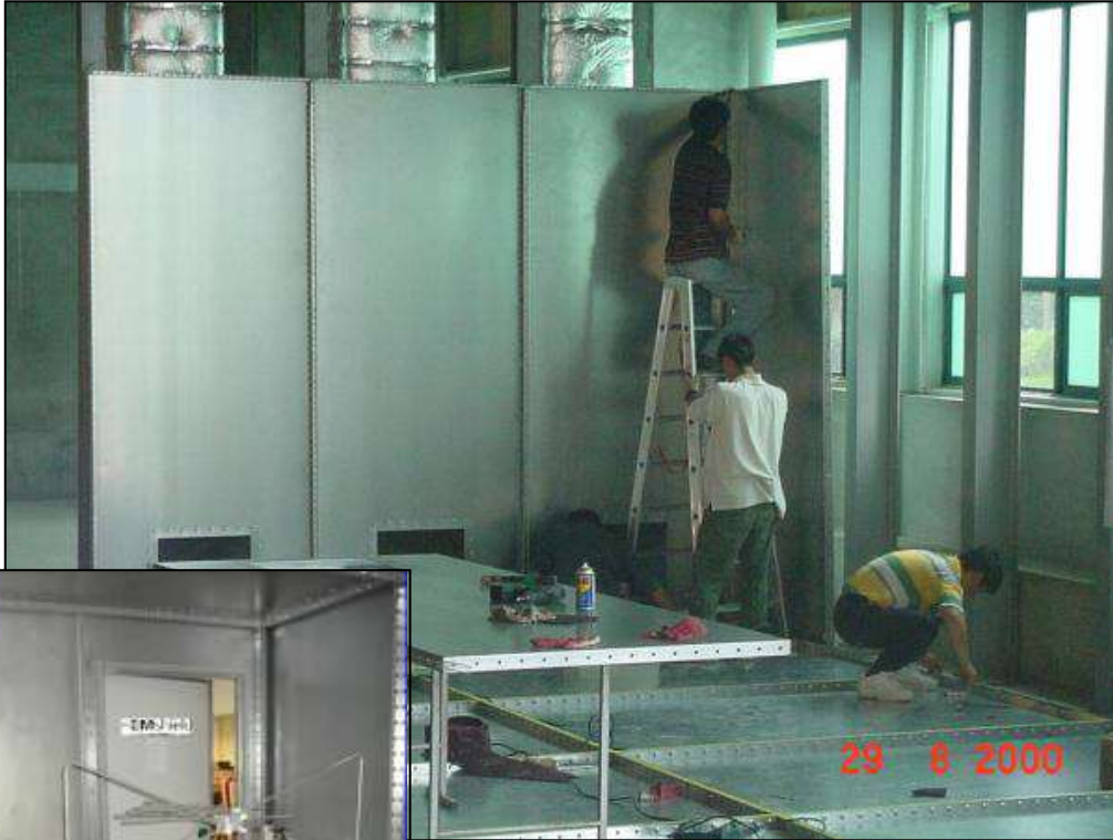
Installation inside normal building
